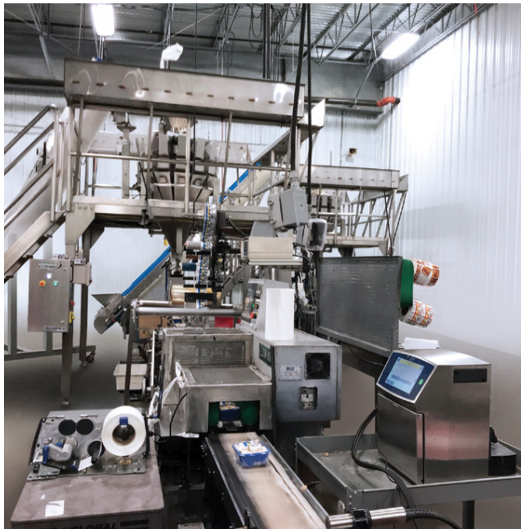
J-M Farms' new combination scale anchors an all new primary packaging line with conveyors, hoppers, labelers, metal detection, and more.
