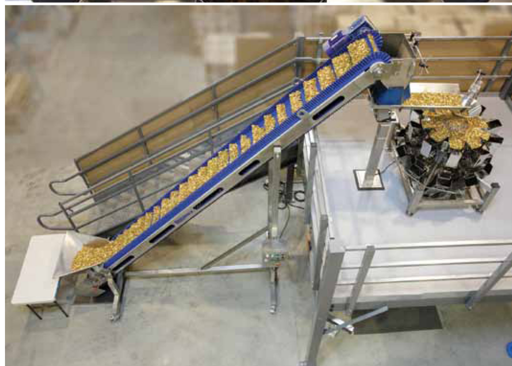
A food-grade incline conveyor system transfers raw product to the top of the mezzanine level prior to being dumped into the 10-head PrimoWeigher 360 bucket scale below.
